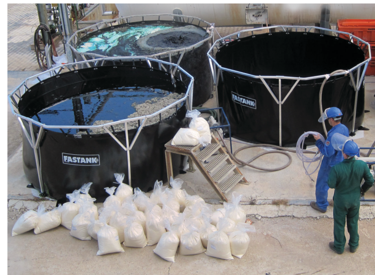
Overhead view of the metal recovery operation, including portable treatment tanks and Smopex® fibre ready to be charged.
